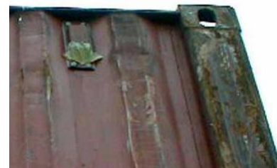
Figure 5.20 Vent tapped over
