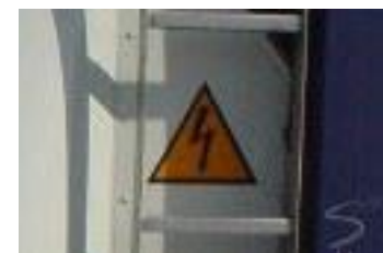
Figure 8.5 Overhead warning sign
