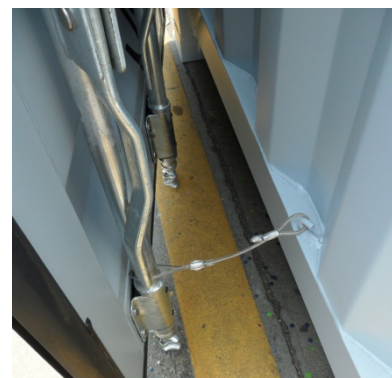
Figure 5.30 Door retaining strap
