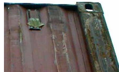
Figure 5.20 Vent tapped over
